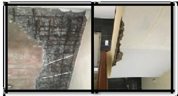
Figure 25: Spalling and Corrosion
