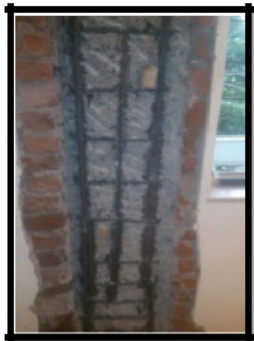
Figure 1: Corrossion in Rebars
