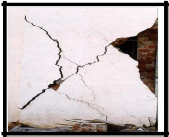
Figure 15: Visible Spalling of Concrete
