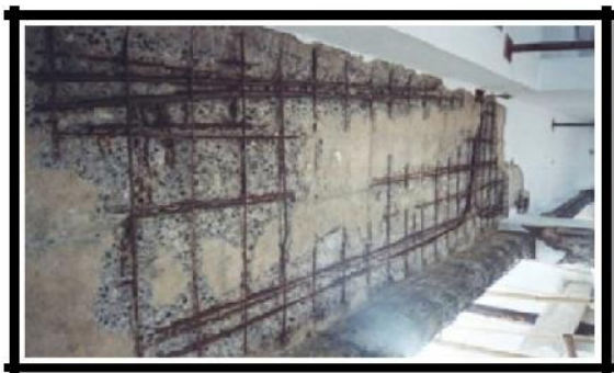
Figure 16: Corrosion of Exposed Reinforcement
