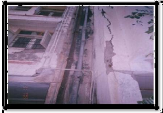
Figure 19: Vertical Cracks Along Concrete Cover Line
