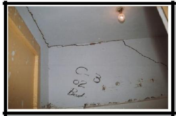
Figure 21: Cracks After Earthquake
