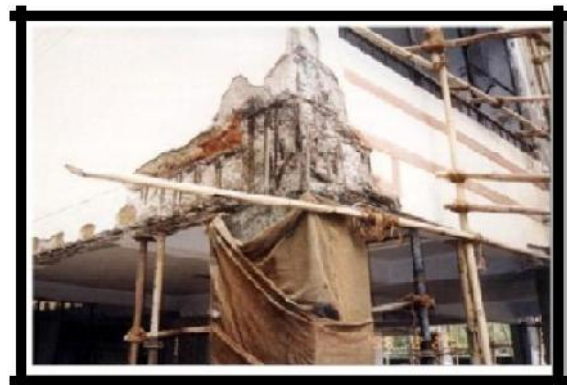
Figure 17: Corrosion of Rebars at Joints
